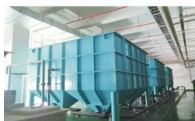
Backwash and Accumulation Factory
