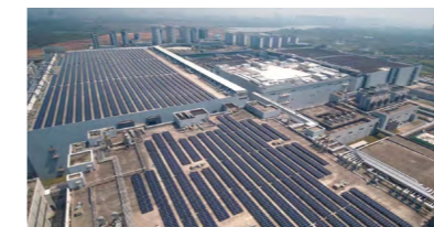
Rooftop PV Solar Systems at Wuhan CSOT
