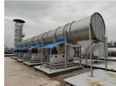
VOC Activated Carbon Adsorption Tower of Huizhou CSOT
